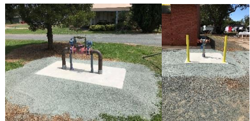
Fire hydrant and hose reel at Elmore Caravan Park
